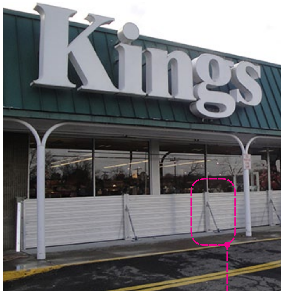
1. Manual flood shields deployed
